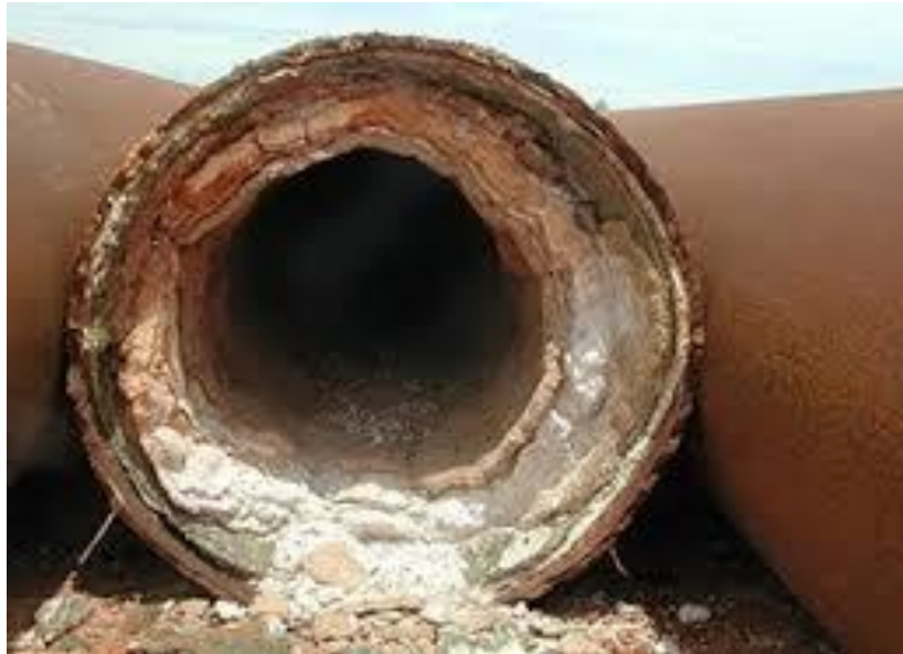
Figure 01: Scales formed inside the Pipe
